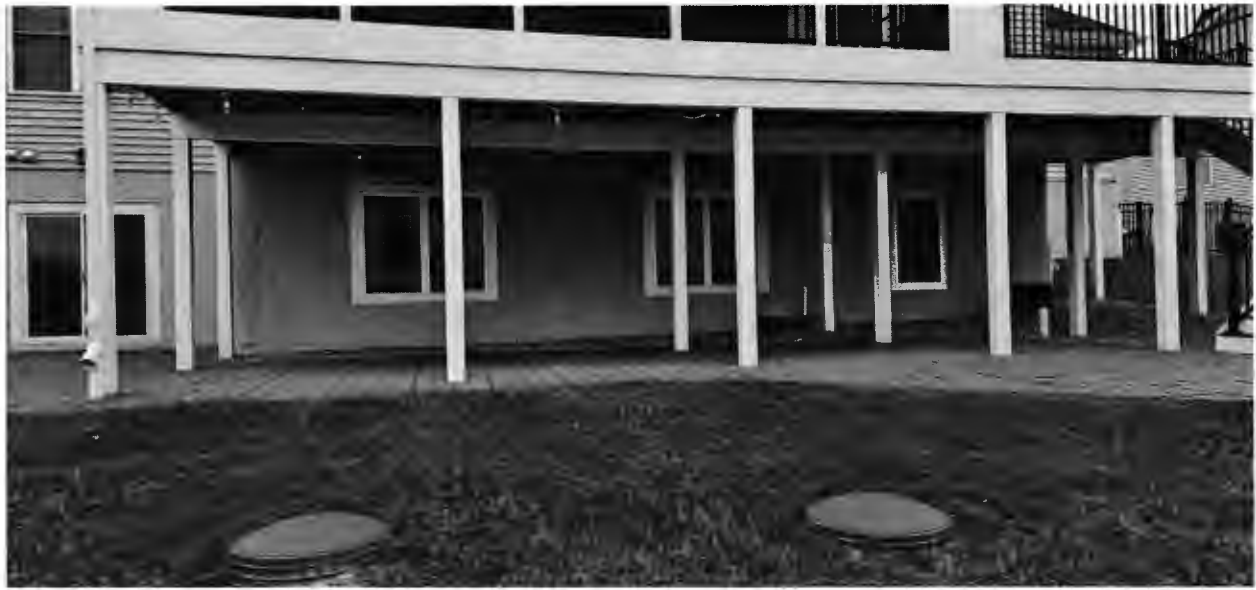
Septic Tank Manhole Covers
