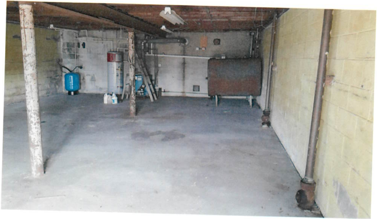
Basement parcel 1. Two septic stacks along the rear wall and one in the corner near the oil tank.
