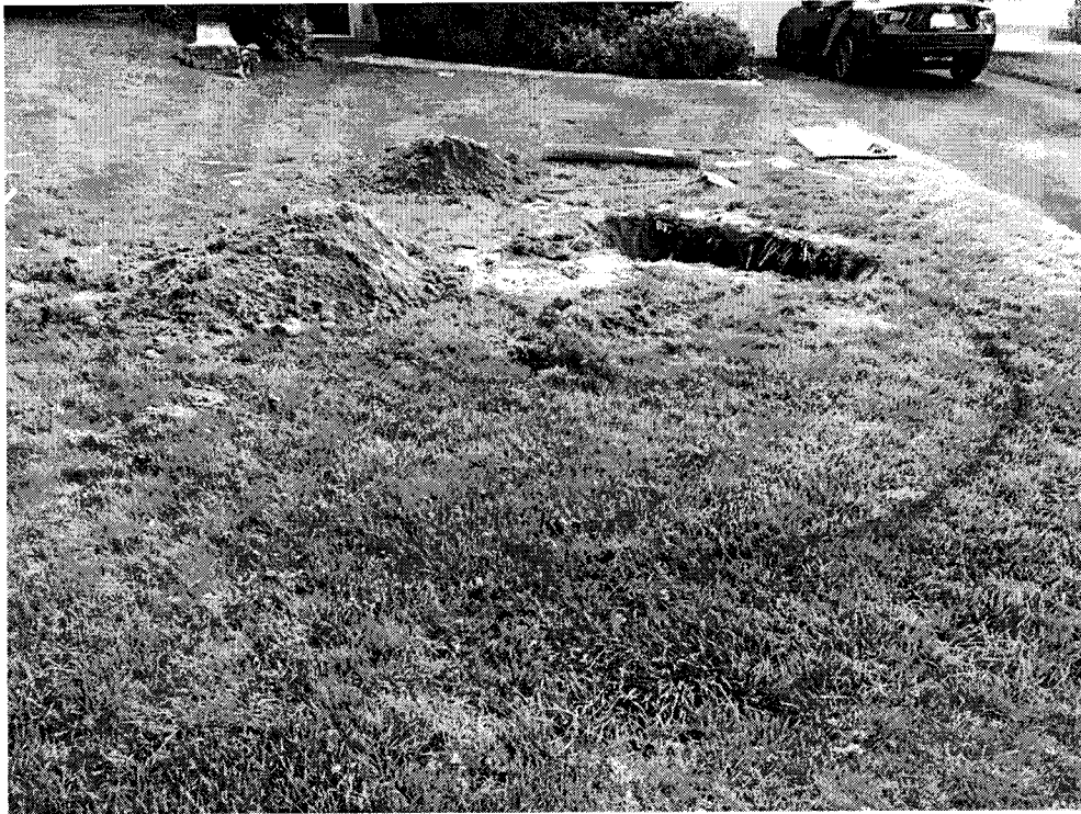
Red ring shows limits of dry well (note depression in foreground at perimeter)
