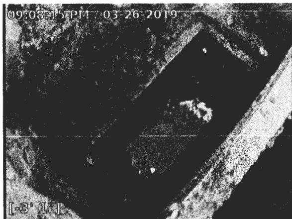
3/26/2019 9:08:15 PM Shows an excavated distribution box was used to introduce the camera into each of the drainfield lines. Shows there to be 3 drainfield outlets in the excavated distribution box.
