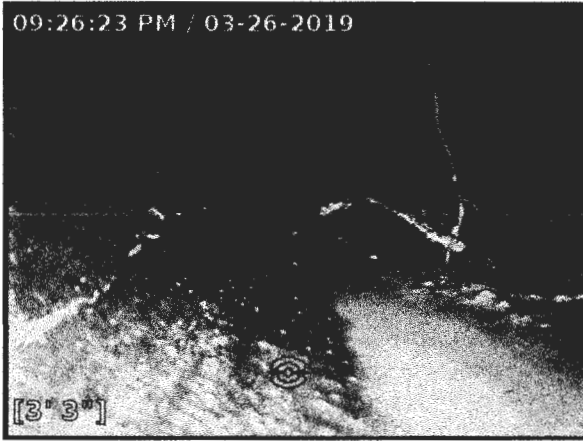
3/26/2019 9:26:23 PM 3' 3" Shows a break in the line in solid portion of line in drainfield line B. This will need to be remediated by a license contractor.
