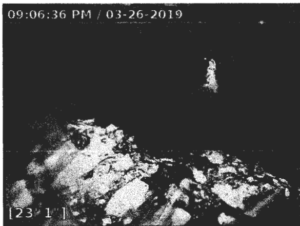
3/26/2019 9:06:36 PM 23' 2" End of the PVC back line. Shows the inside of the distribution box. The camera was advanced from this point in the PVC back line back towards the septic tank.
