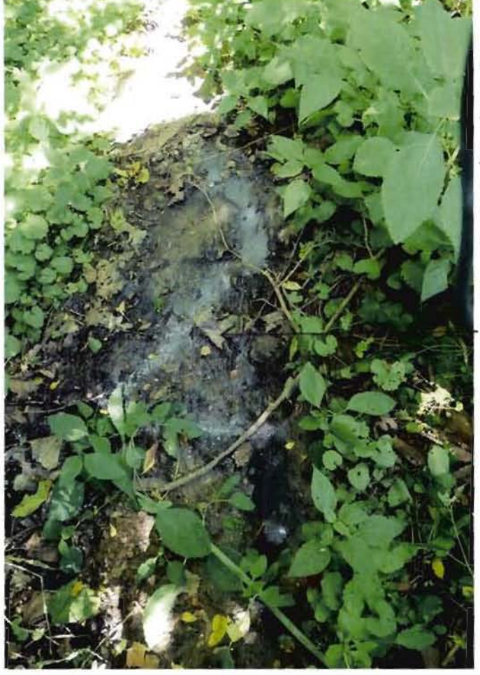
Discharge occurring on backside of property behind shed.
